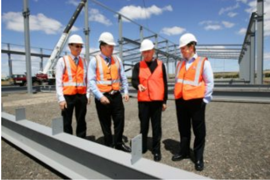
MAJOR PROJECT: Project co-ordinator Richard Bisinella, MP Richard Marles, director Lino Bisinella and RPC's Andrew Sarich at the site
